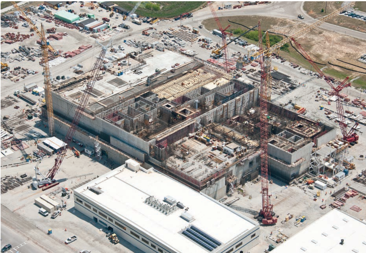
MOX Fuel Fabrication Facility under construction at the Savannah River Site in South Carolina, 2012.
